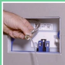
Flush water supply
